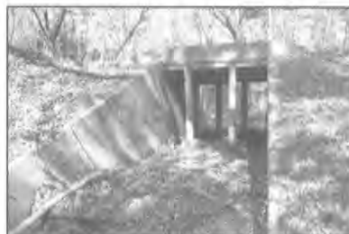
Waste Weir Overflow
