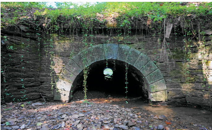
Many travelers never notice the intricate infrastructure, such as this culvert that is under the canal.
