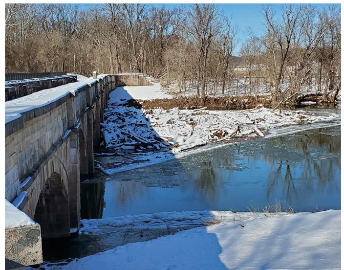
Debris build-up at Monocacy Aqueduct – Photo by Jon Wolz
