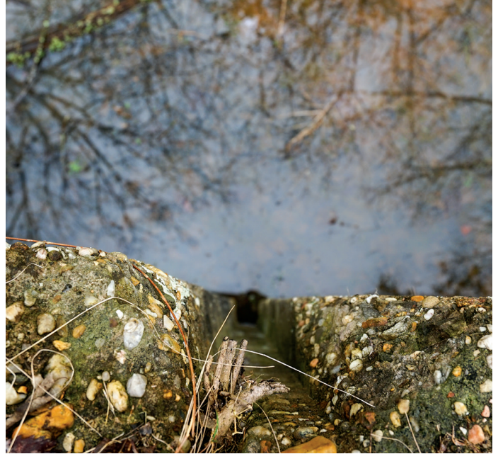
Plank slot in a stop gate
