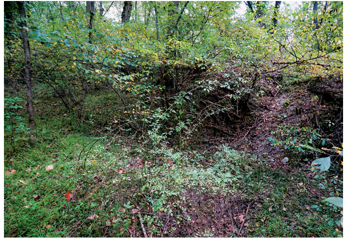
Sinkhole in the canal prism close to McCoy's Ferry
