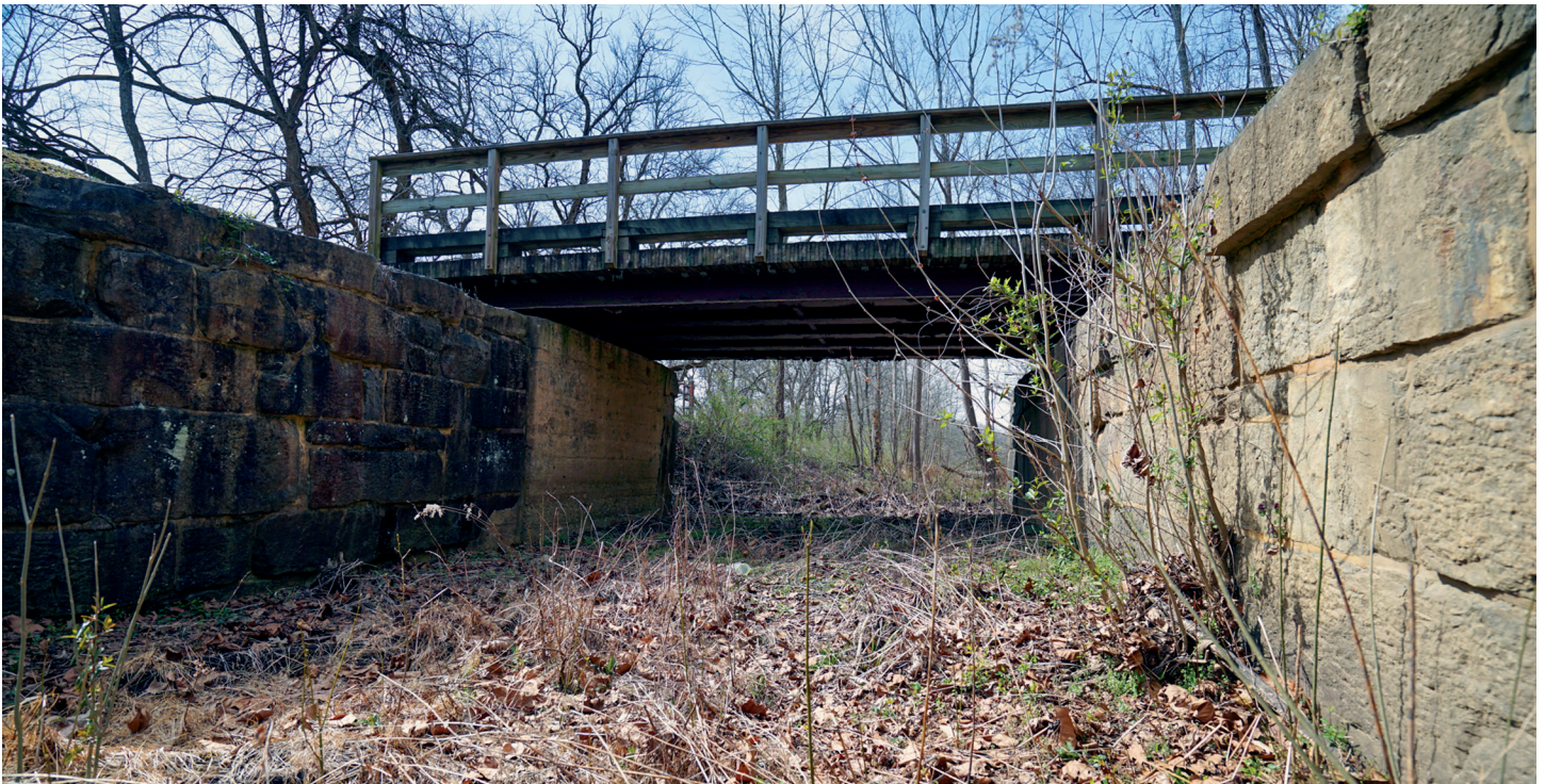
Stop gate at east end of Big Pool. There was a drop gate here as well as the mounting foundations for a swing bridge. The swing bridge remains are at the west end of the gate.
