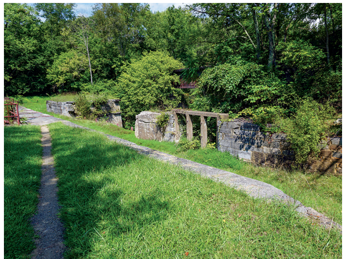
Waste weir built into the berm side in an aqueduct superstructure. In this case the water was drained into the creek that the aqueduct crossed.
