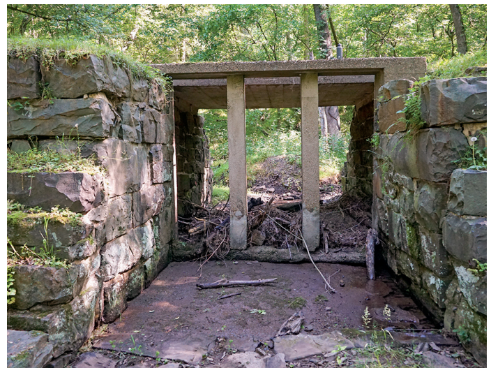
Waste weir exit side with concrete replacement gate and bridge and original stone work on the walls.
