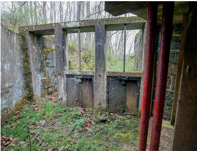
Butterfly gates in the bottom of a waste weir. The modern steel supports under the bridge portion are visible in the foreground.
