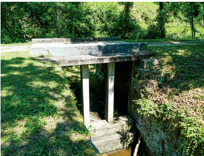
A typical waste weir on a sunny day.
