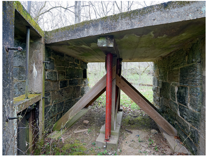
Timber and steel supports reinforcing the later concrete bridge replacement. Note that the original stone support walls were retained.
