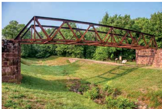
The remnants of the iron bridge at Whites Ferry.
