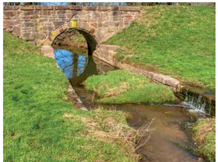
Culvert 51 at Whites Ferry is easily observed from the towpath. It had a wooden trunk and prism floor – Photos by Steven Dean
