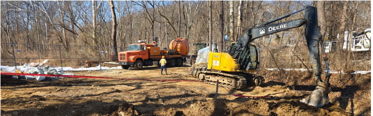
An earthen dam under construction above Lock 10. Photos above and below by Allyson Miller
