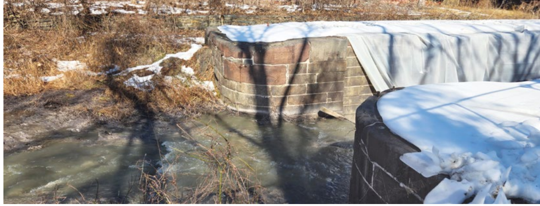
(Left) Cofferdam at Lock 13; sludge and debris collecting around vegetation in canal prism; sewage flowing into canal below Lock 12. (Right) Lock 13 with plastic sheeting displaced. All photos by Allyson Miller
