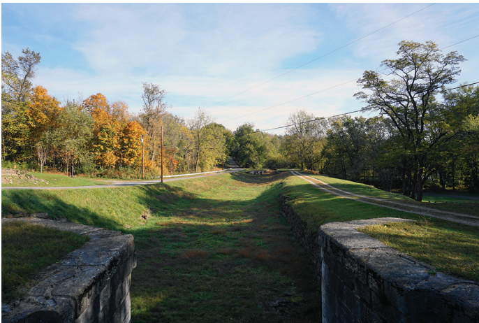
View from lock 49 looking east. Construction of Lock 47 began in February 1836 and by May 1839 all four locks were completed.
