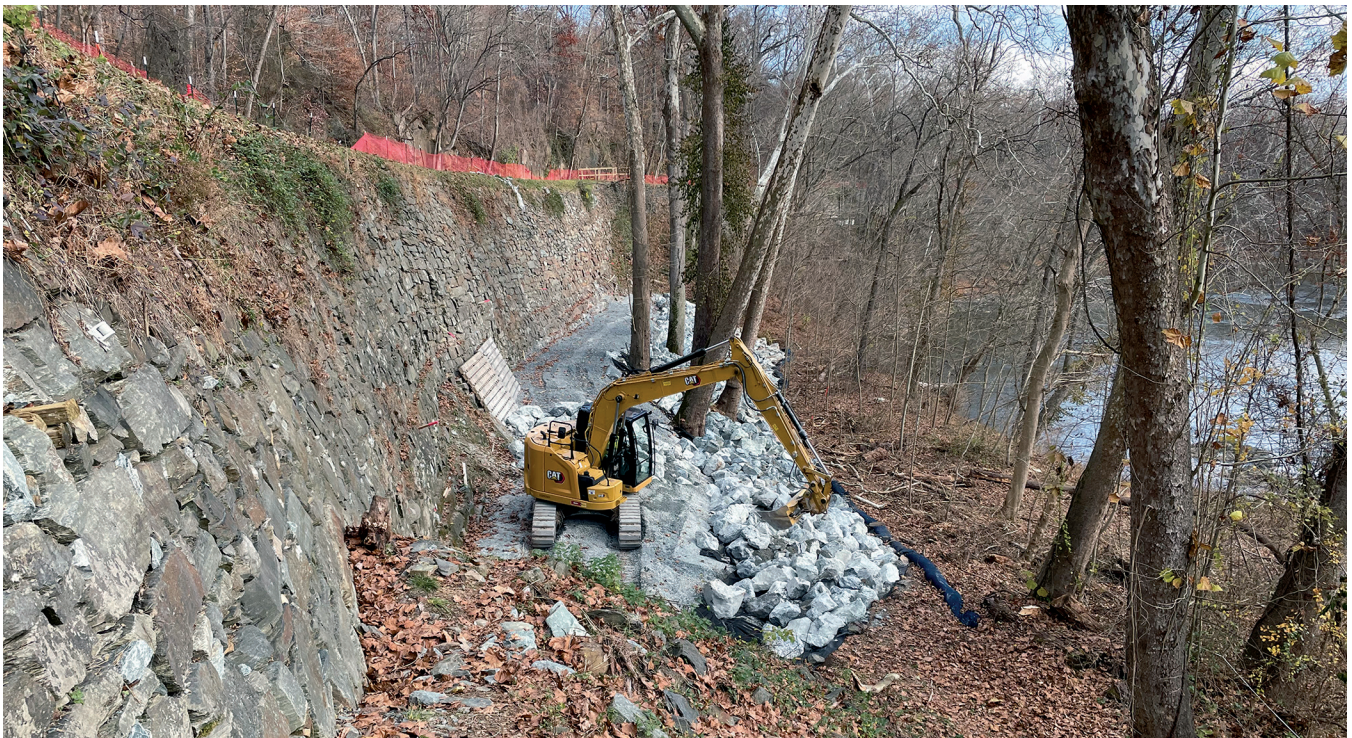
The building of the Log Wall upstream riprap buttress – Photo by C&O Canal NHP Professional Services Division
