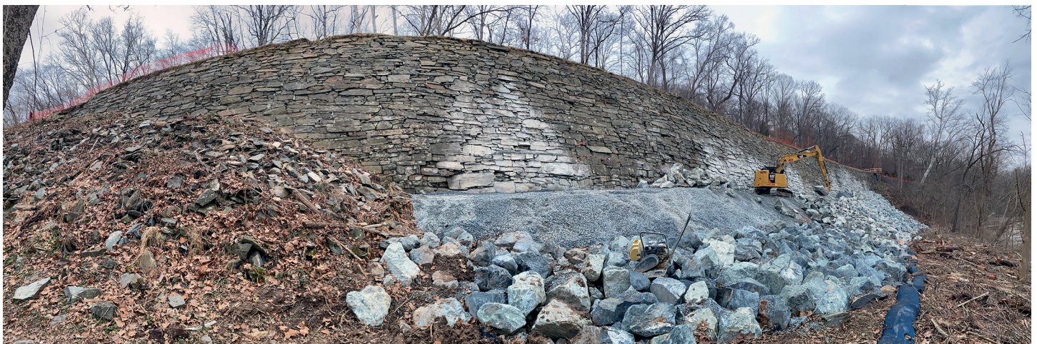
Panorama view of the construction of the upstream buttress – Photo by C&O Canal Professional Services Division
