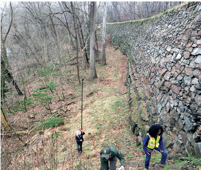
A 2020 upstream view of Log Wall before project work began – Photo by C&O Canal Professional Services Division
