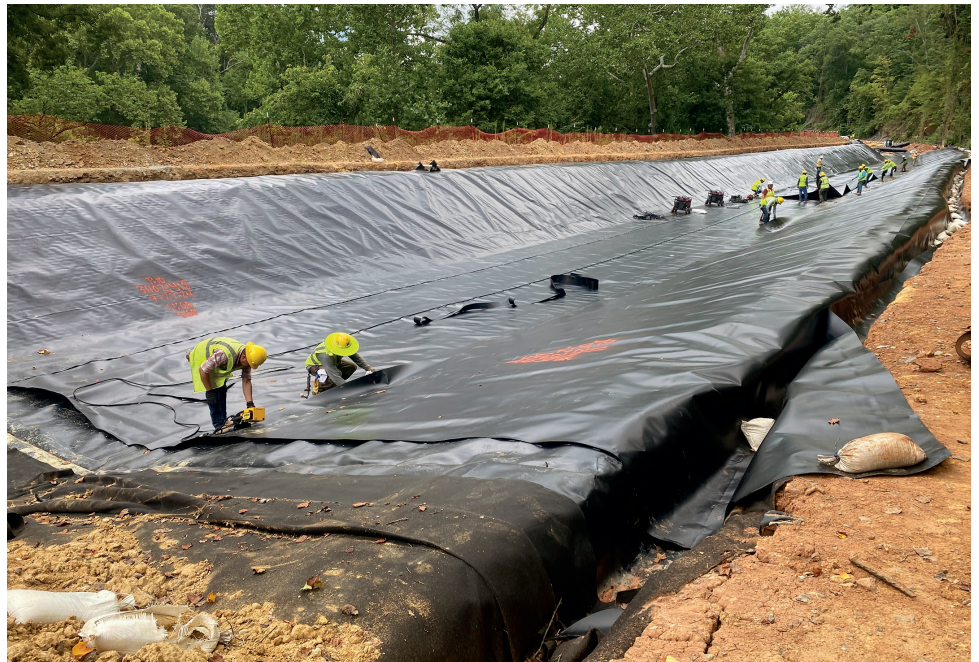
The installation of the canal prism liner – Photo by C&O Canal Professional Services Division
