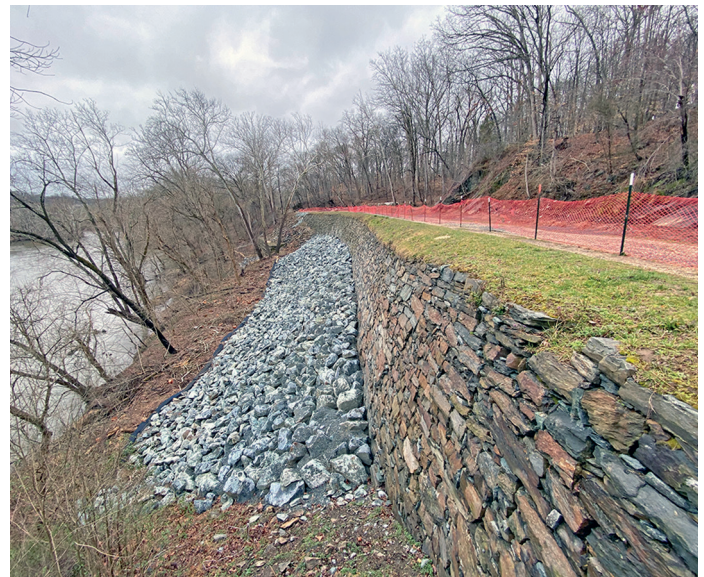
A March 2024 upstream view of Log Wall after repairs – Photo by C&O Canal Professional Services Division
