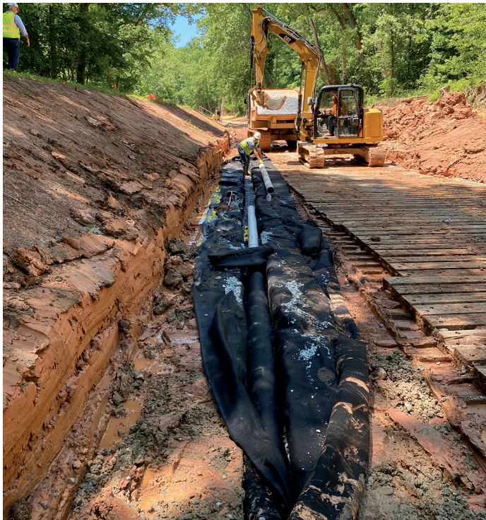
The installation of an underdrain system within the canal prism – Photo by C&O Canal Professional Services Division
