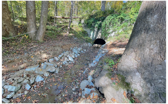
The stabilization of a tributary leading into the canal prism – Photo by C&O Canal Professional Services Division
